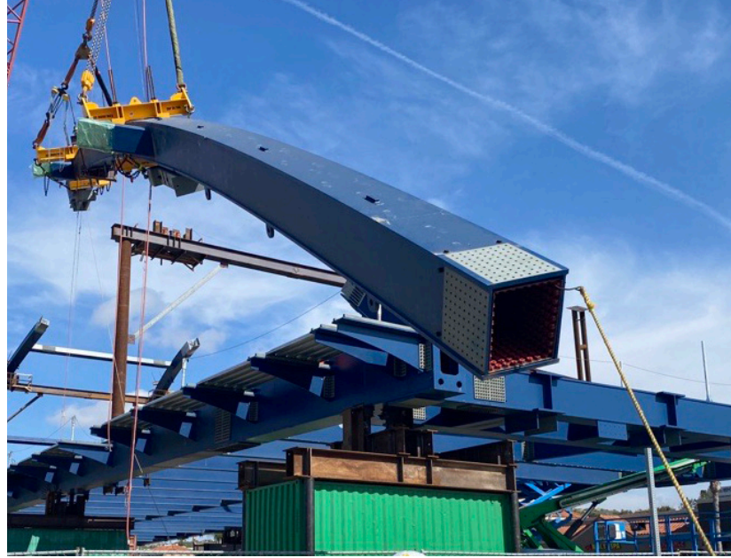
An arch rib with Shuriken being lifted into place. Walsh prepared complex rigging to lift the tilted arch ribs in the proper orientation.
