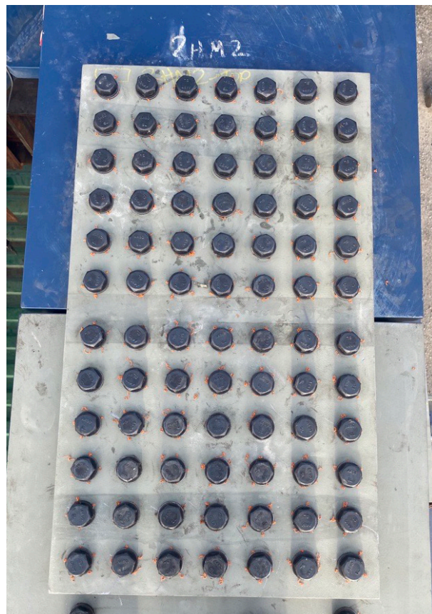
[TOP] Support diaphragms being set for connections to the tie girder using Shuriken. [BELOW] A completed bolted splice using Shuriken. The orange media from DuraSquirt DTI washers helped crews and inspectors verify that the bolts are tight.
