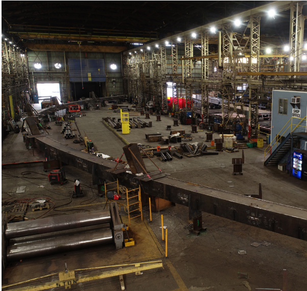
HSS22x22x7/8 stubs being set for attachment to the built-up arch ribs. The inclined ribs made for complex geometry with tight tolerances.
