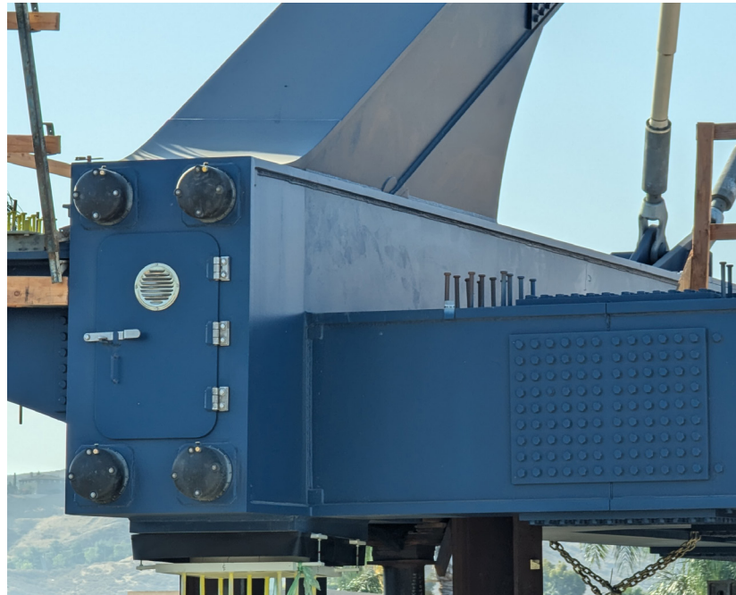
A “knuckle” of the bridge, where a support diaphragm, arch rib, and tie girder come together. The anchorages for the four post tensioned cables are visible.
